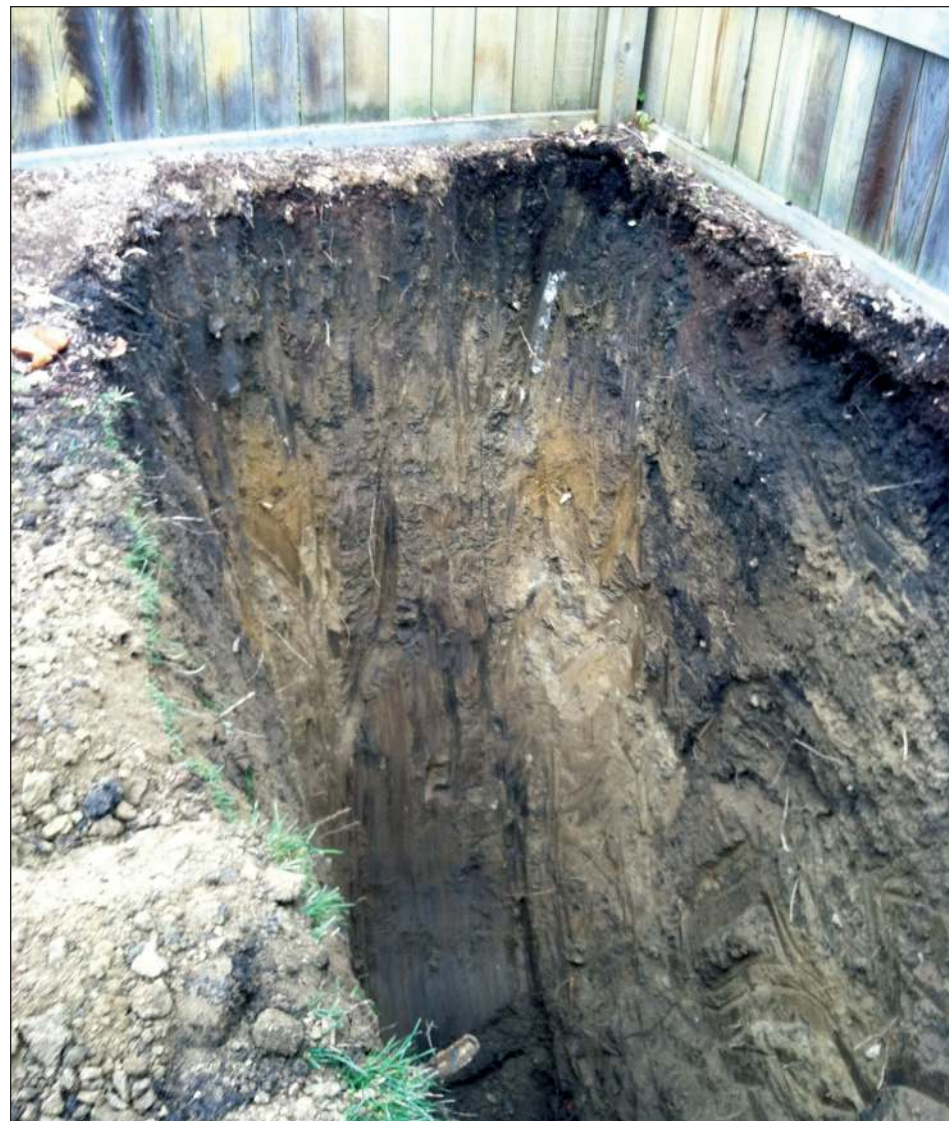
Twelve-foot deep hole needed for sanitary sewer repair in a resident's backyard.
