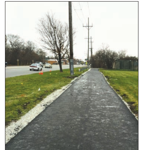
New bike path constructed along the north side of Cermak, between Mannheim and Westchester Blvd.
